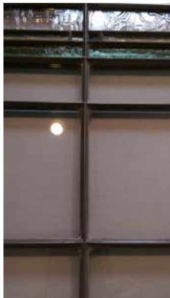
This detail of zinc coming on a conserved window shows the clean solder joints of experienced glass artists.
